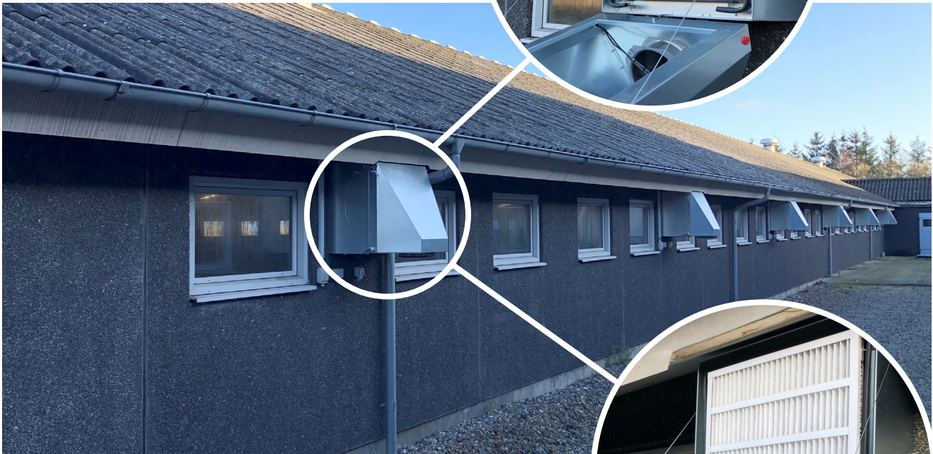
Hatting barn with newly installed filtration housings.
